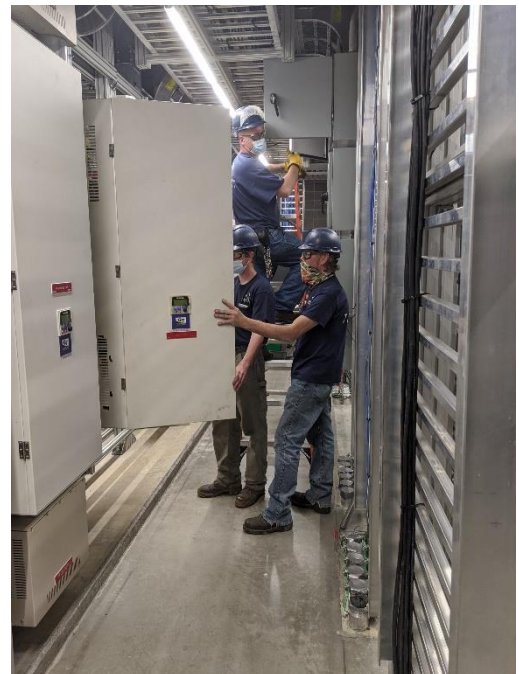
Lynden Nelson, Kyle Lamprecht, and John Sackett working on a drive for an ammonia compressor
