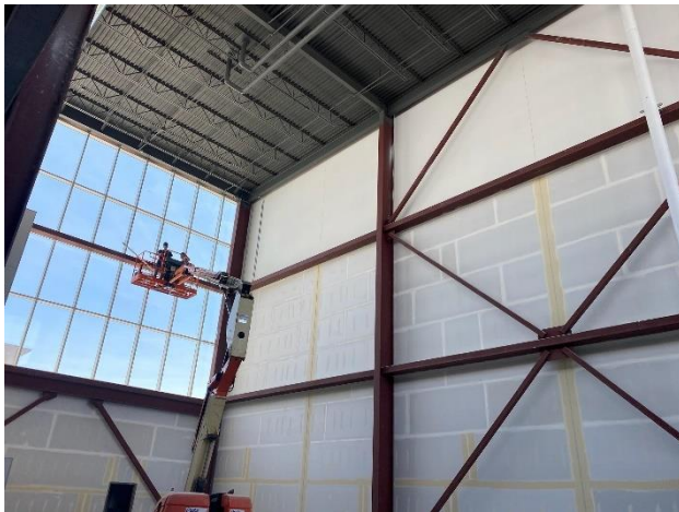
Brock Linafelter and Chad Peters running conduit for powered curtains in the rock-climbing area
