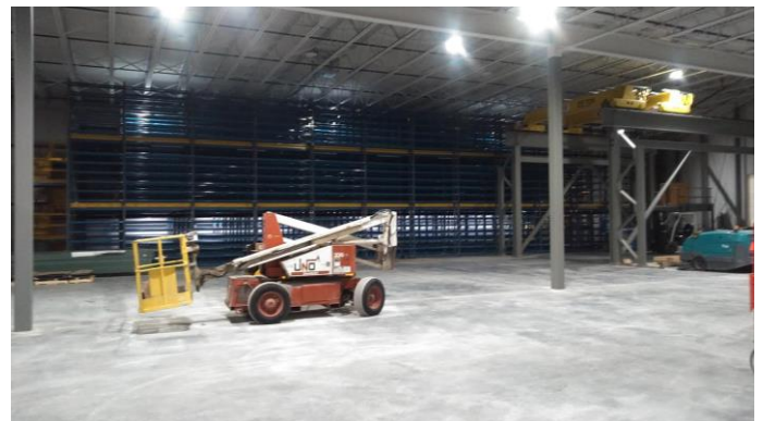
Assembly parts rack lighting
