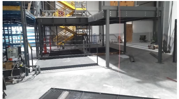
Parts rack lift and mezzanine
